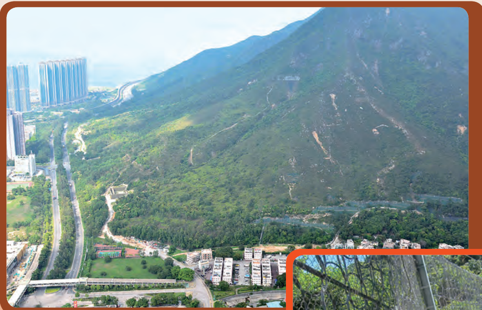
東涌壩尾的天然山坡山泥傾瀉災害緩減措施（柔性防護網） Natural terrain landslide hazard mitigation measures in Pa Mei, Tung Chung (flexible barrier)
