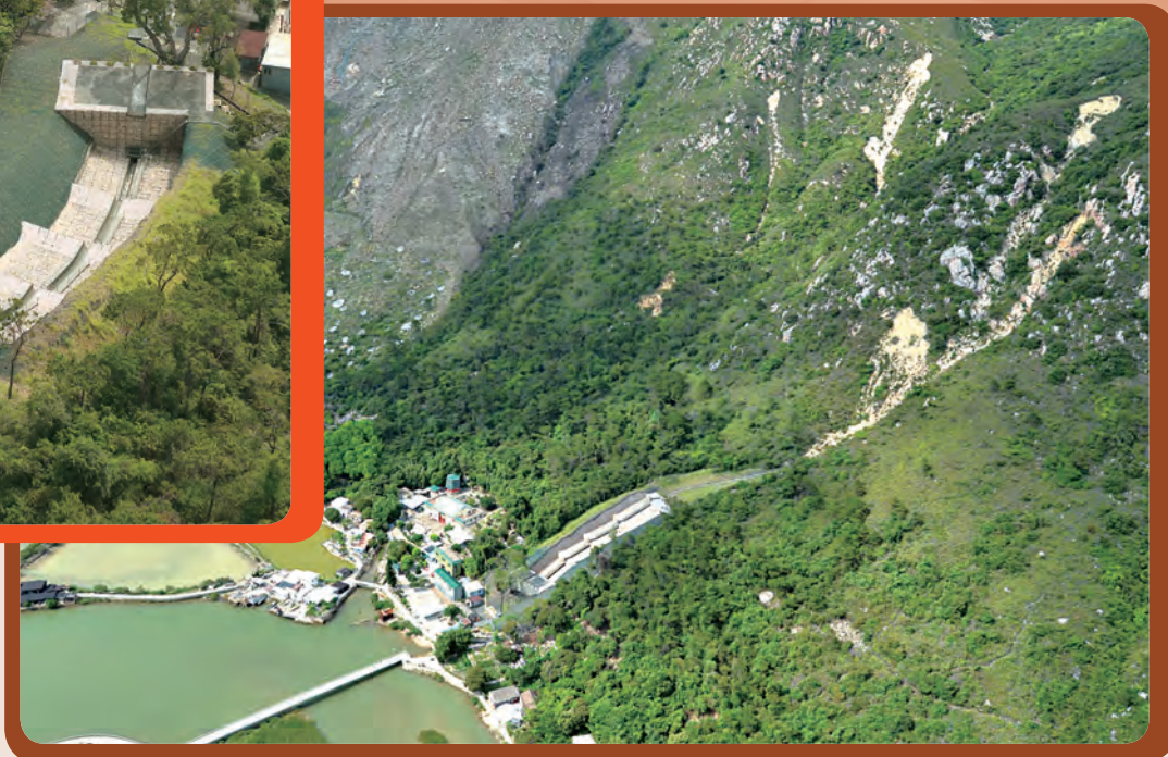
大澳南涌的天然山坡山泥傾瀉災害緩減措施（石籠泥石壩） Natural terrain landslide hazard mitigation measures in Nam Chung, Tai O (gabion barrier)
